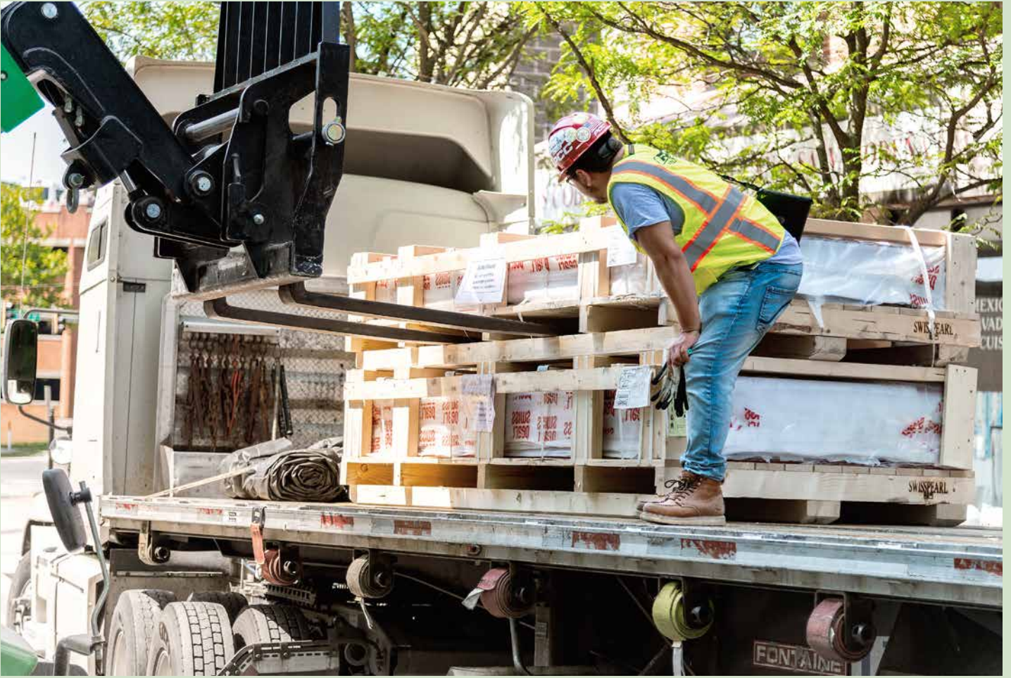
10 At the port of arrival, the Swisspearl pallets are again loaded onto a truck.
