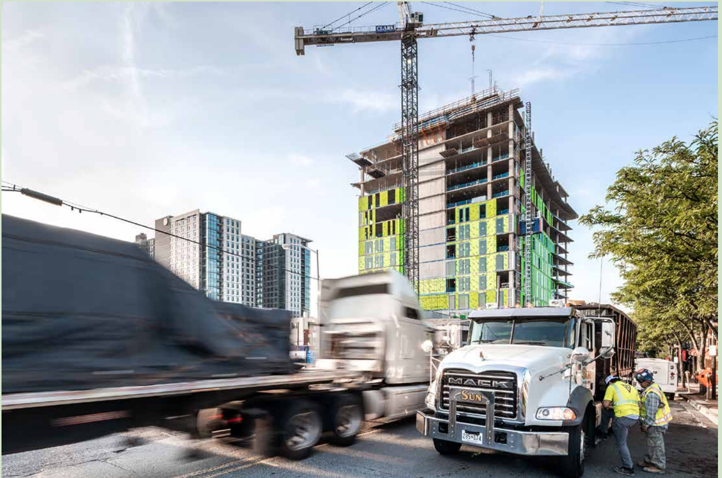
12 After their delivery to the building site in Gaithersburg (Maryland), the assembly of the panels directly from the palettes occurs as quickly as possible.
